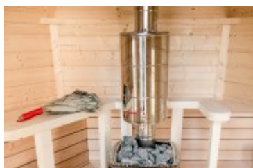
Water Tank For Woodburning Heaters
