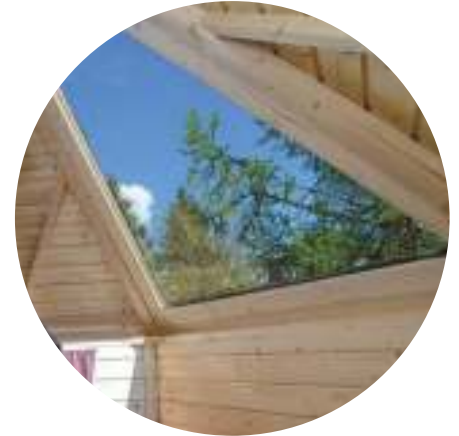
Roof window is not opening. The glass is clean and tempered, 8 mm thick
